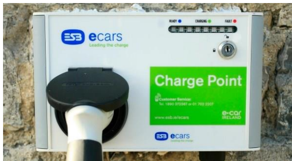
Figure 10.1 Electric Car Charging Points
