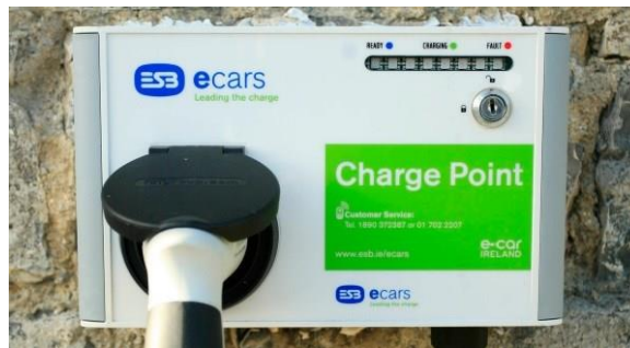
Figure 10.1 Electric Car Charging Points
